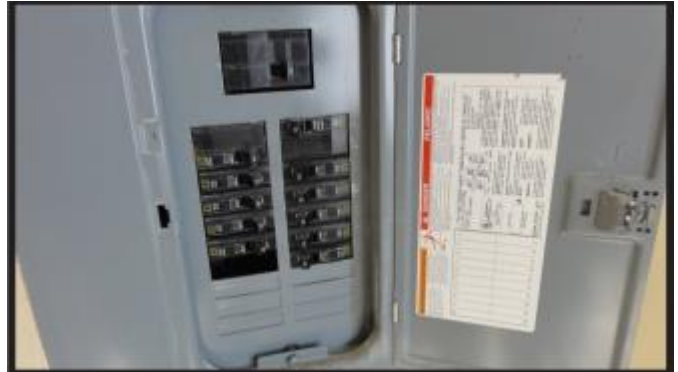
An Example of an: Electrical Box/Panel
