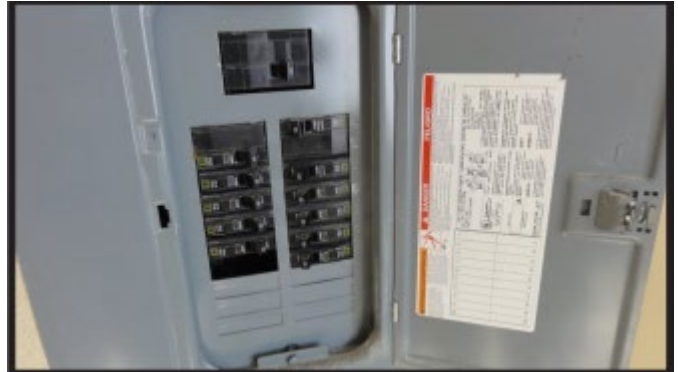
An Example of an: Electrical Box/Panel
